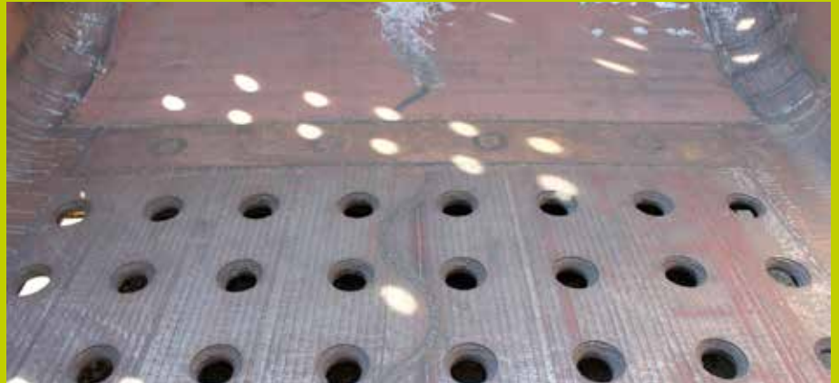
Duroxite® plates welded together with the gaps properly filled between liners to prevent spalling.
