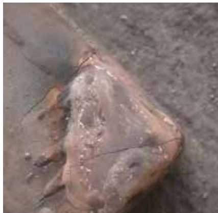
Thicker overlay is welded away from the corner, thinner overlay at the edge.
